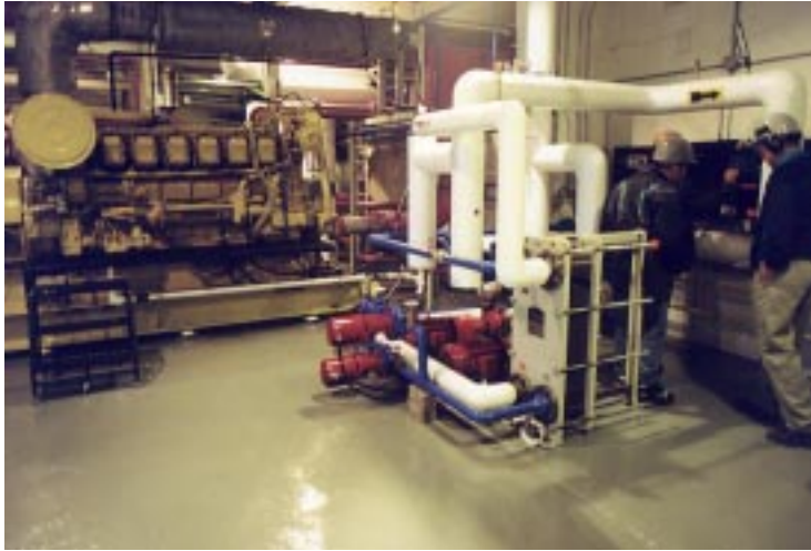
Reducing dependency on imported fuels, cutting environmental impact and lowering heating cost is the goal of residual heat recovery systems like this one in Fort McPherson. Based on this initial project design in 1996, residual heat upgrades and new systems have been commissioned in three more communities in the past two years.
