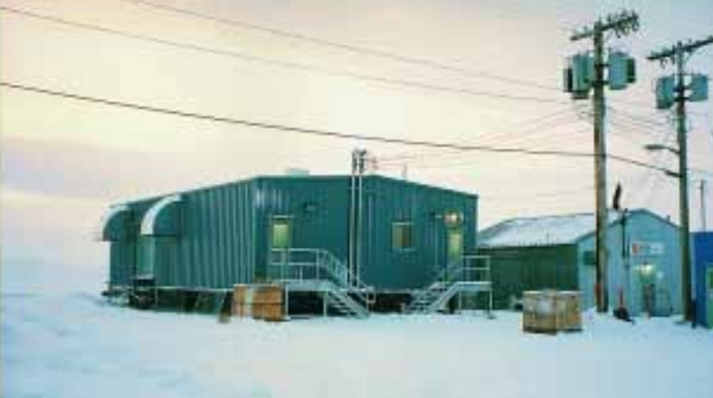
A new modular power plant was completed in Paulatuk during the past year.
